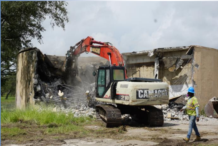
The old round city water tank at Deberry and Lamont is now down. This project was part of the City's ongoing community clean-up/demolition program.
